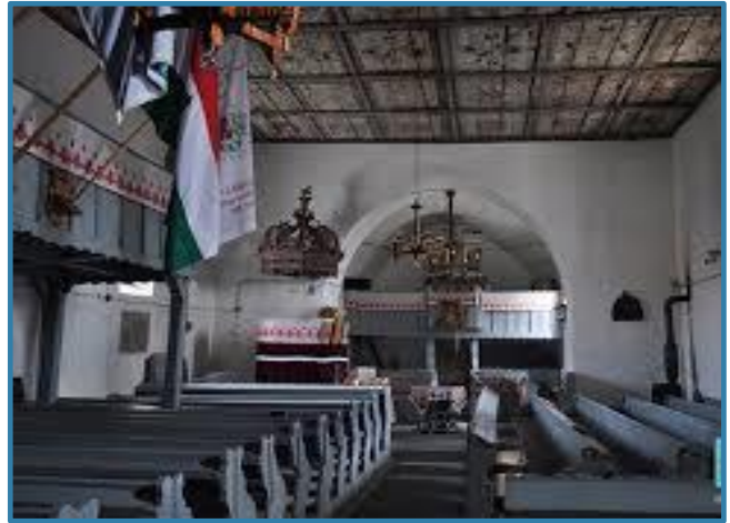
The Nyárádszentmárton church is undergoing restoration from damage caused by the communist regime in the 1990's.
